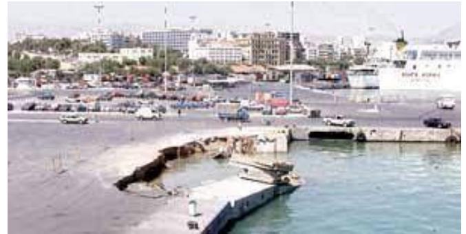
Figure 1. The collapsed quay wall.
