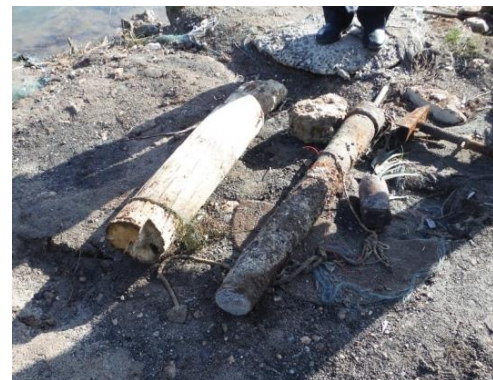
Photo 3. Clearly cut of wooden and steel column.
